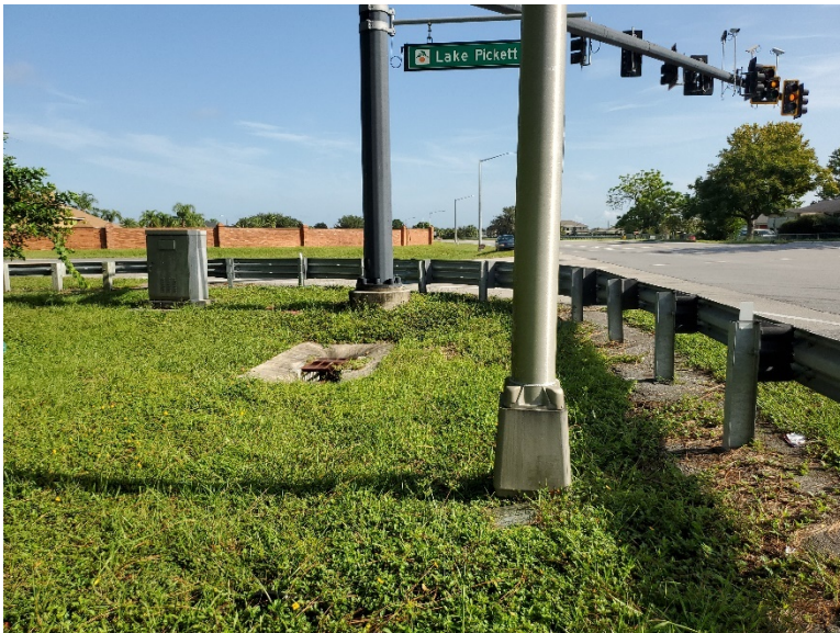
Ditch bottom inlet at southwest intersection of Lake Pickett Road and Chuluota Road, facing north.
