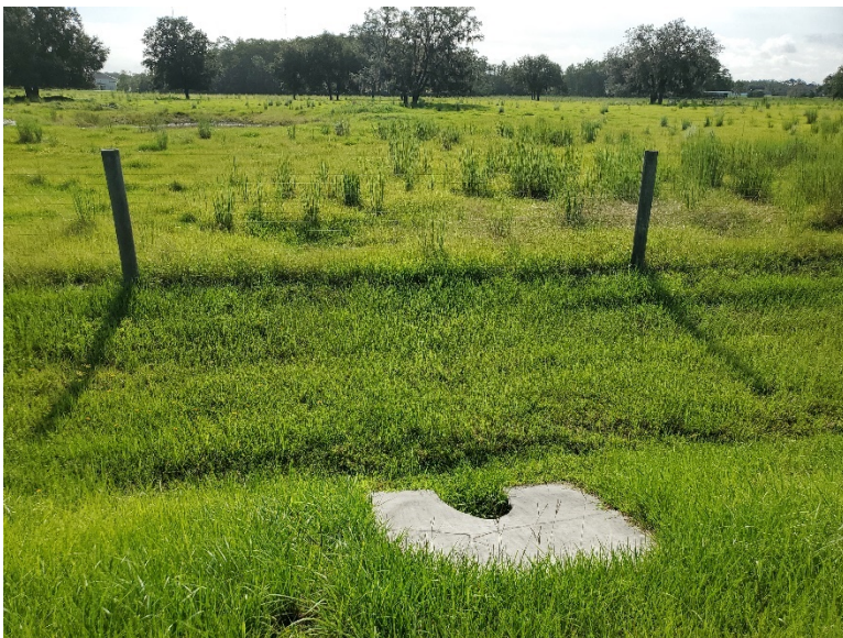
Existing inlet which conveys offsite runoff from pasture to existing storm drain along Chuluota Road, facing east.
