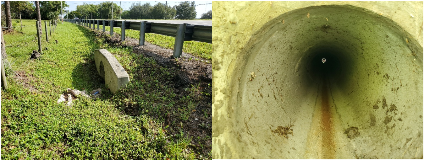
Cross drain which conveys runoff from basin 4-300 to storm drain on east side of Chuluota Road, facing north and east.
